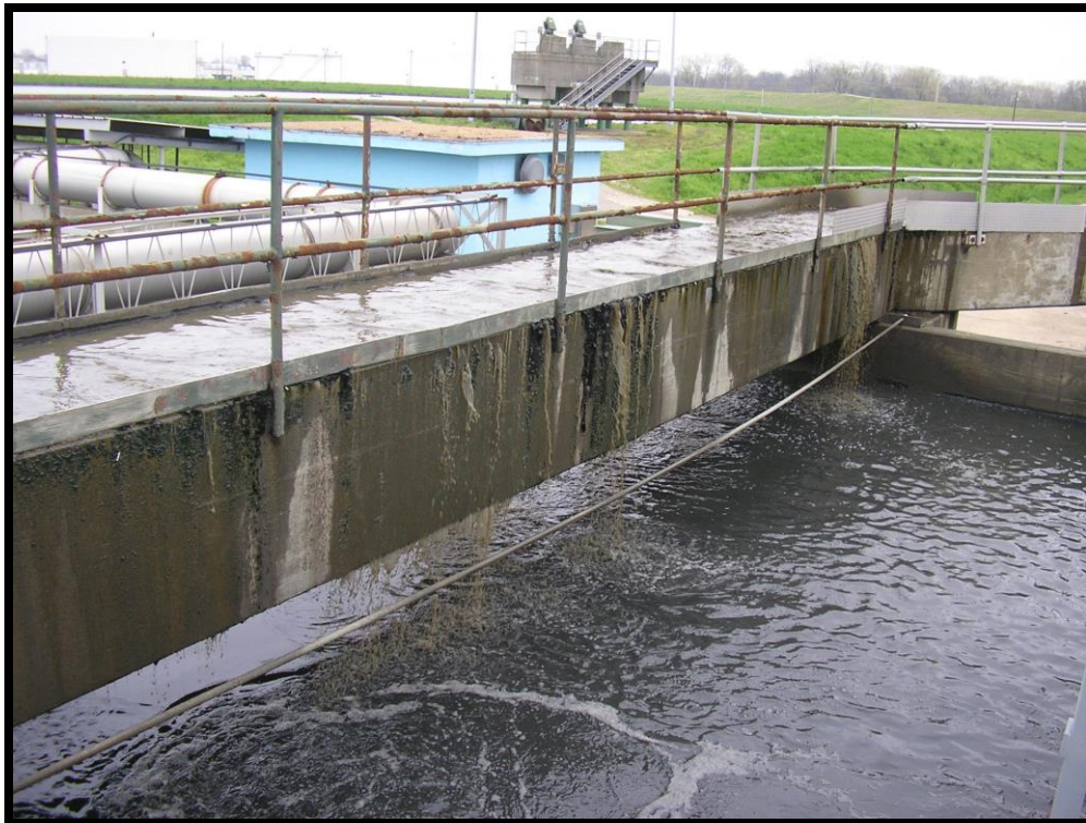
Overflowing condition of Flow Distribution Channel Immediately Downstream of RAS Connection
