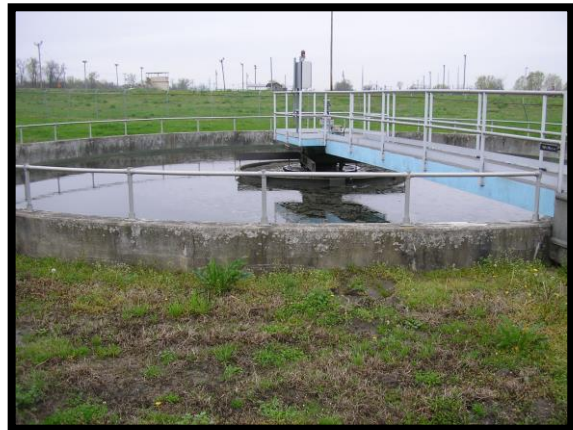
View of Center Fed Clarifier
