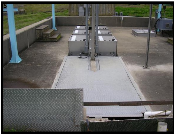
Existing UV Channel and Equipment
