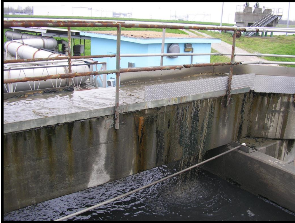
Overtopping of Influent Channel at Head of Aeration Basins
